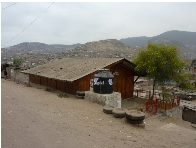
After four years the roof needs to be redone
